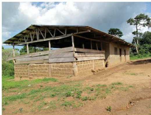
Figure 2: Condition of a disadvantaged school building
